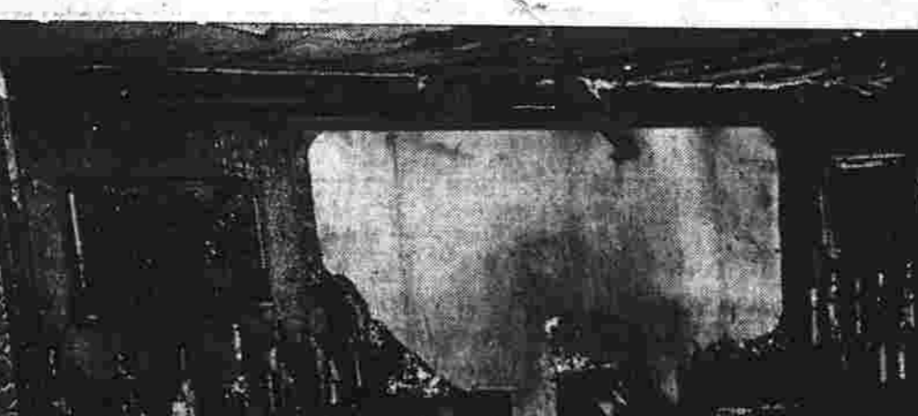
The barroom was one of the most heavily damaged areas.
